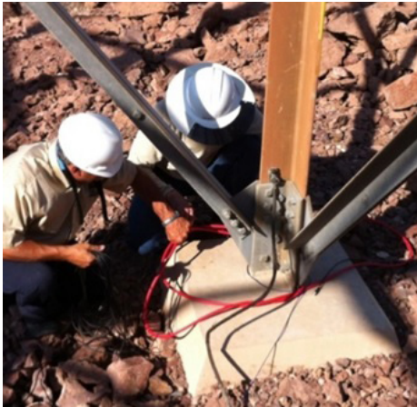
Installing the GroundFlex® probes (in this illustration, the probes are looped twice around the tower leg)
